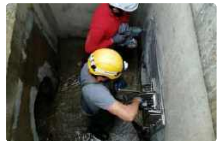
Installation VHA Ilot
